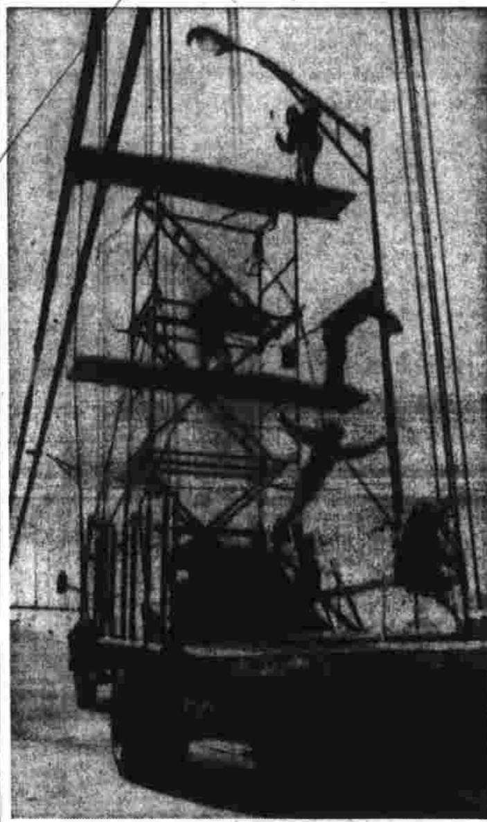
Bridge Painting Ballet Working from scaffolding mounted on a truck, painters strike ballet-like poses as they put finishing touches on the Verrazano-Narrows Bridge, scheduled for opening Nov. 21. The bridge, across the entrance to the New York harbor, connects Brooklyn and Staten Island. The $525 million structure will be the world's longest suspension span. (AP Photofax.)
